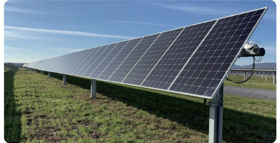
14MW Hy-Grid Solar System
