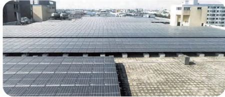
120KW Hy-Grid Solar System In Thailand
