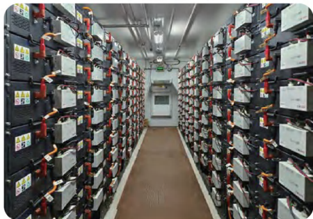
Base station UPS power projects
