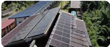
20KW Hy-Grid Solar System In Indonesia
