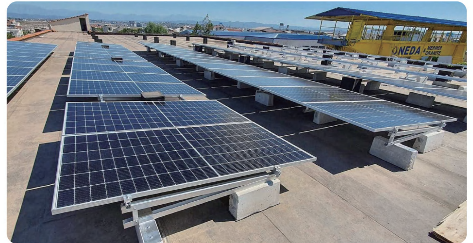
100KW On-grid Solar System in Hungary
